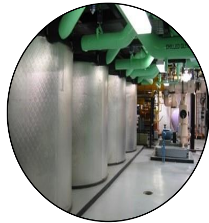
Thermal Energy Storage
